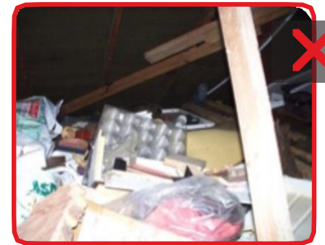
This is not acceptable
